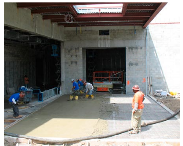
This is our topping slab, at the Daffodil Terrace (an indoor "outdoor" space). Three types of reinforcement were utilized to manage the shrinkage cracking of this thin slab, with no jointing...
